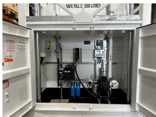
Bunded Lockable Pump Bay
